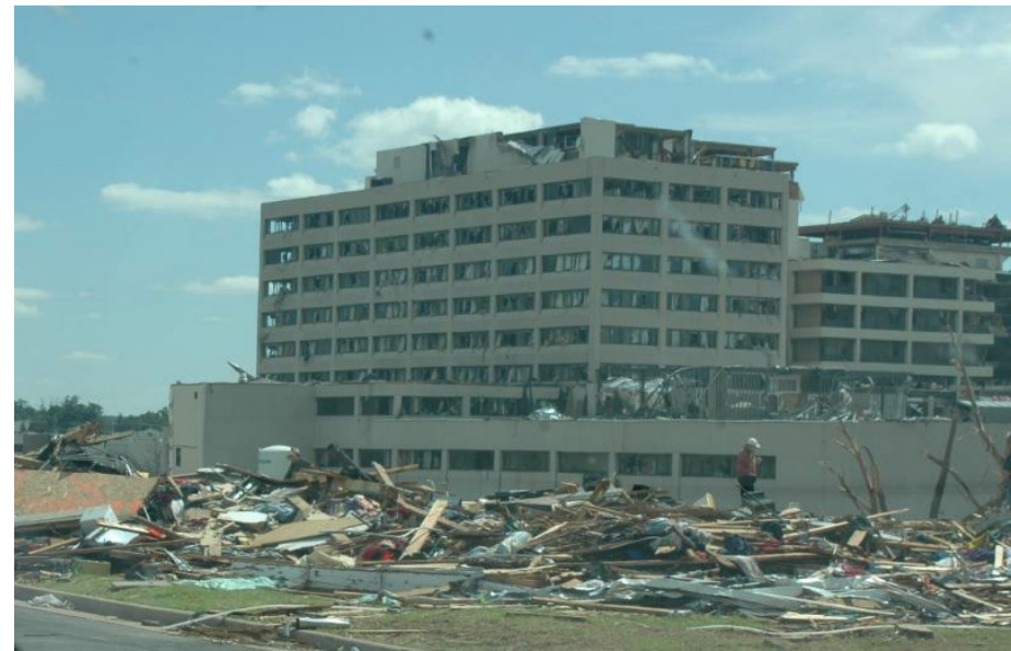
Damage at St. John's Regional Medical Center caused by the May 22, 2011, tornado.
